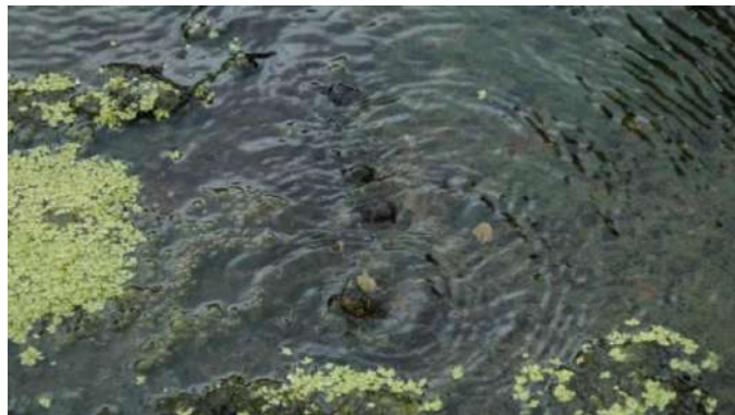
Fig.4 Water gushing from a crack in the pond.
